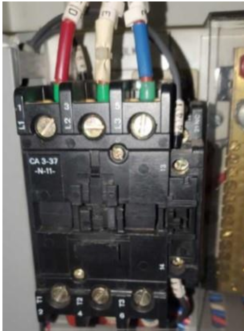
The common main contactor for multiple motor starters which had the white phase contact welded in
