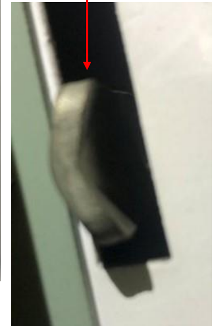
Showing the slot in the metal work between the cell and the cable tier with the door latch tongue in place when door is closed
