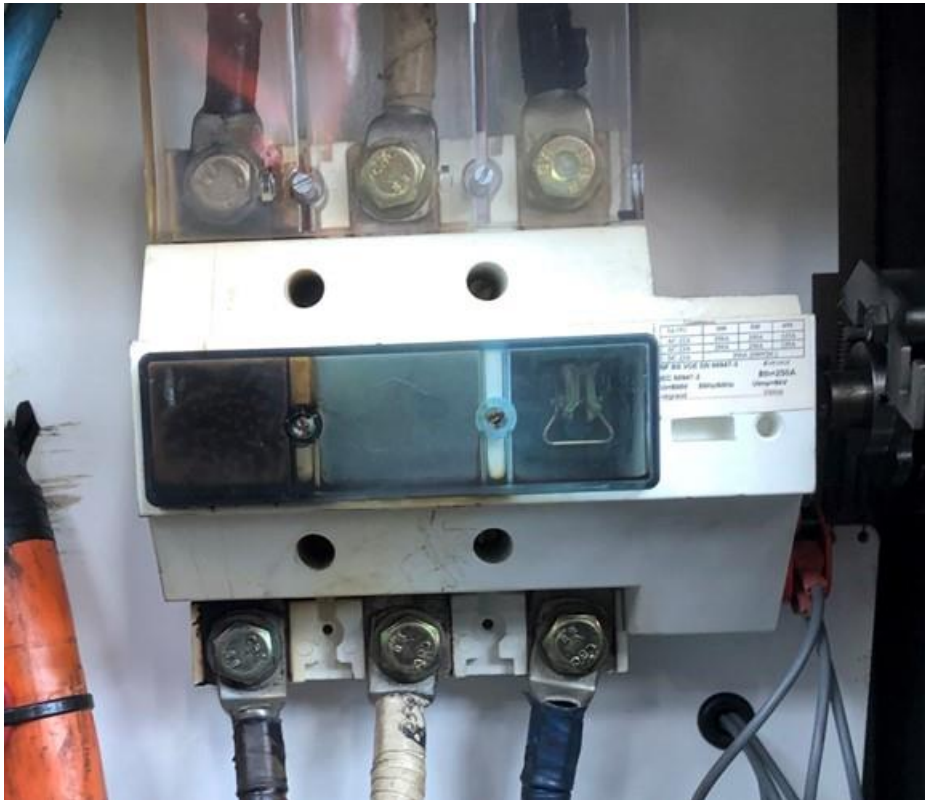
The field isolator contact cover as found.
