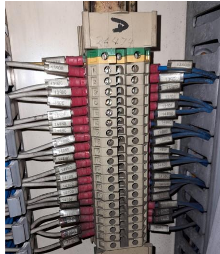
The Regulator panel PLC I/O terminal strip where the redundant cores were terminated.
