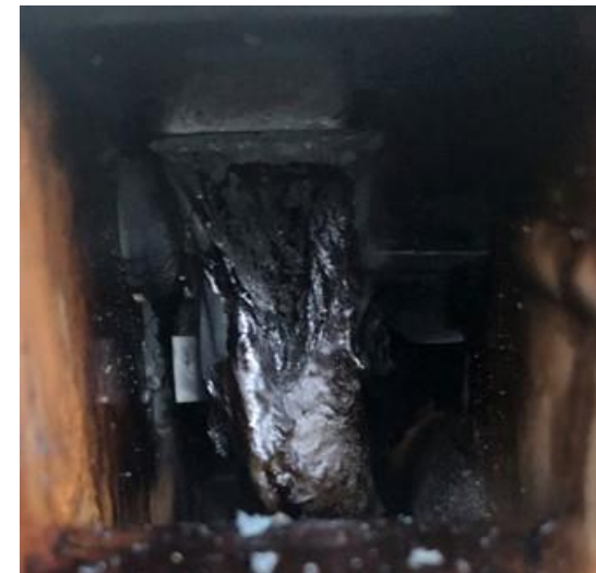
A close up view of the welded red phase contact
