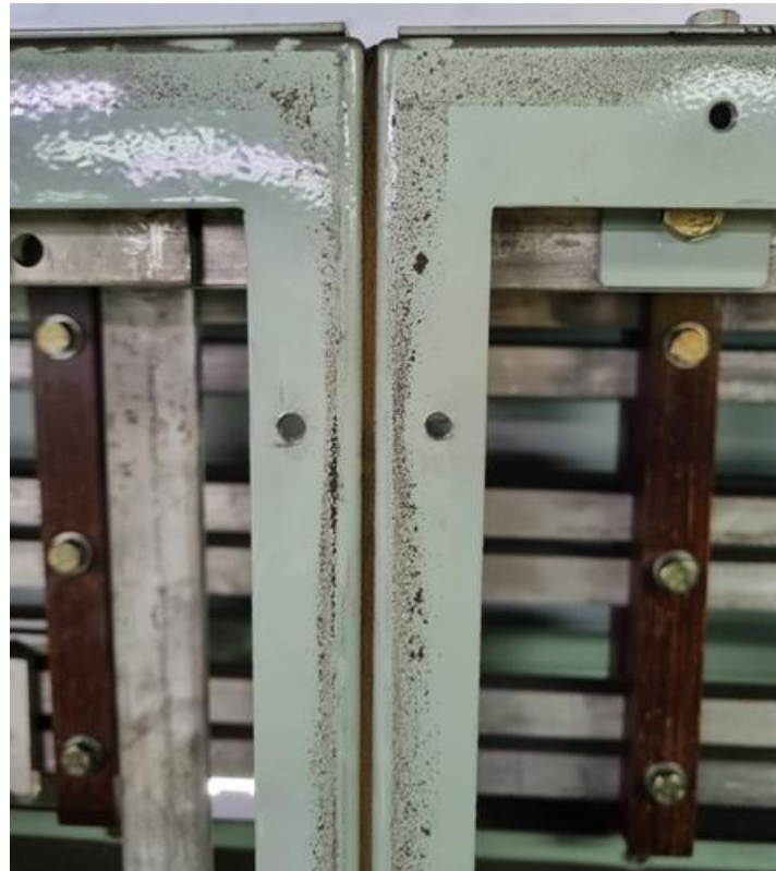
The same gap between the panels as viewed on the side but filled in with appropriate insulation
