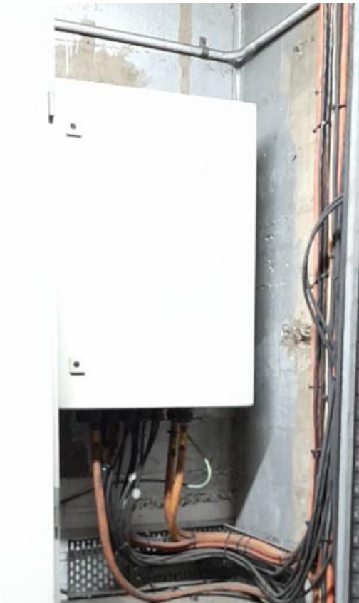
The unknown j-box in the motor room basement where two cables were joined. Note the j-box is not labelled or has an identification and is not mentioned in any of the schematics.
