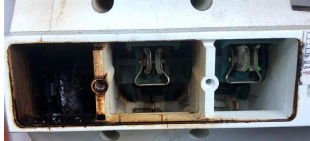
The red phase contact after the plastic cover was removed. The other two phase contacts are still in working order.
