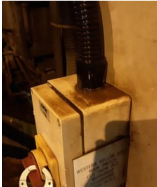
The local isolator with water evident on the top. The top entry cable fitting which has allowed water to ingress onto the isolator contact block.
