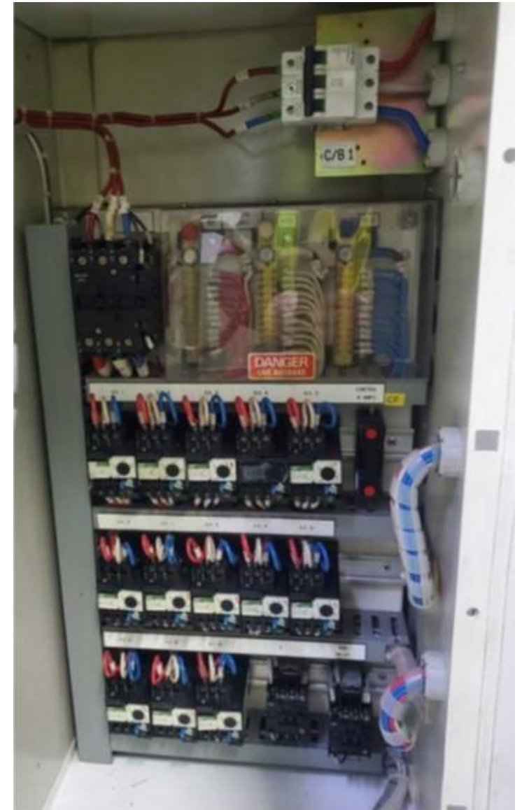
The panel with all the motor starters which has its main isolator on the door
