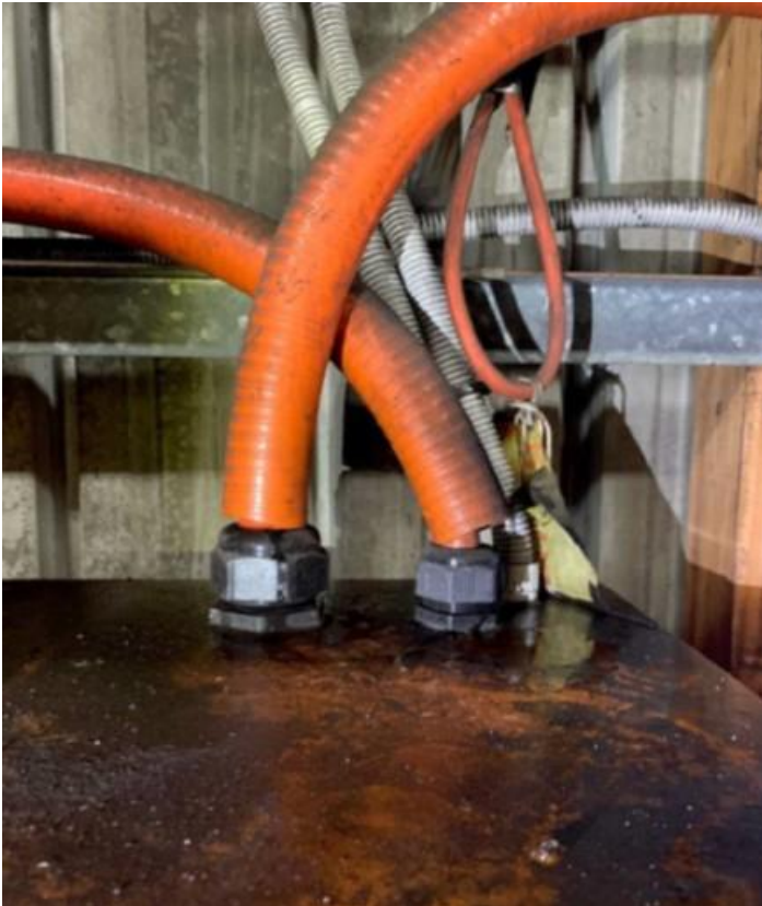
The top of the panel as found covered in water with top entry cables and loosely fitted glands
