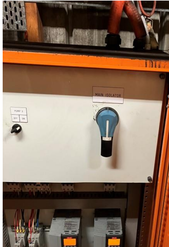
The inside of the panel with the main isolator straight below where the water was entering
