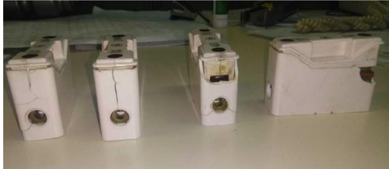
Other neutral link holders with different signs of cracking. Some parts of the holders have broken away exposing the internal conductors.
