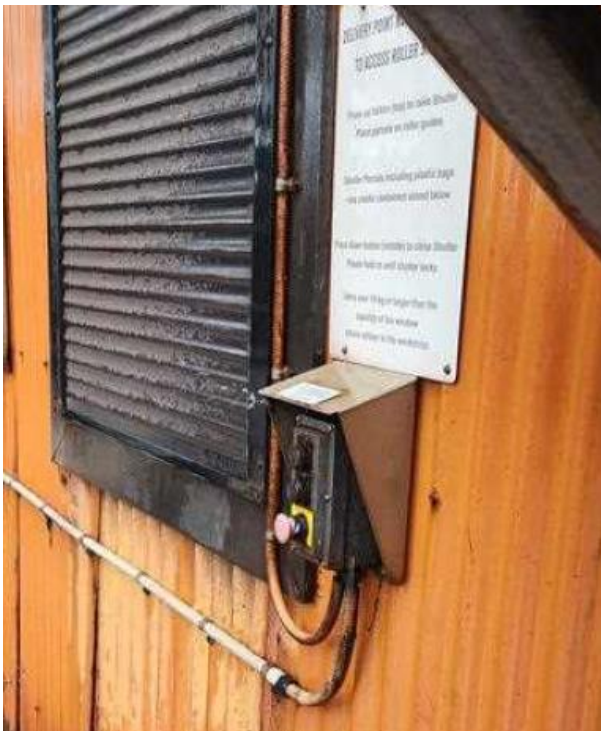
The pushbutton station as found, installed with a weather shroud, IP66 rated enclosure and buttons, bottom entry, compression cable glands and flexible conduit cut off short of the glands.
