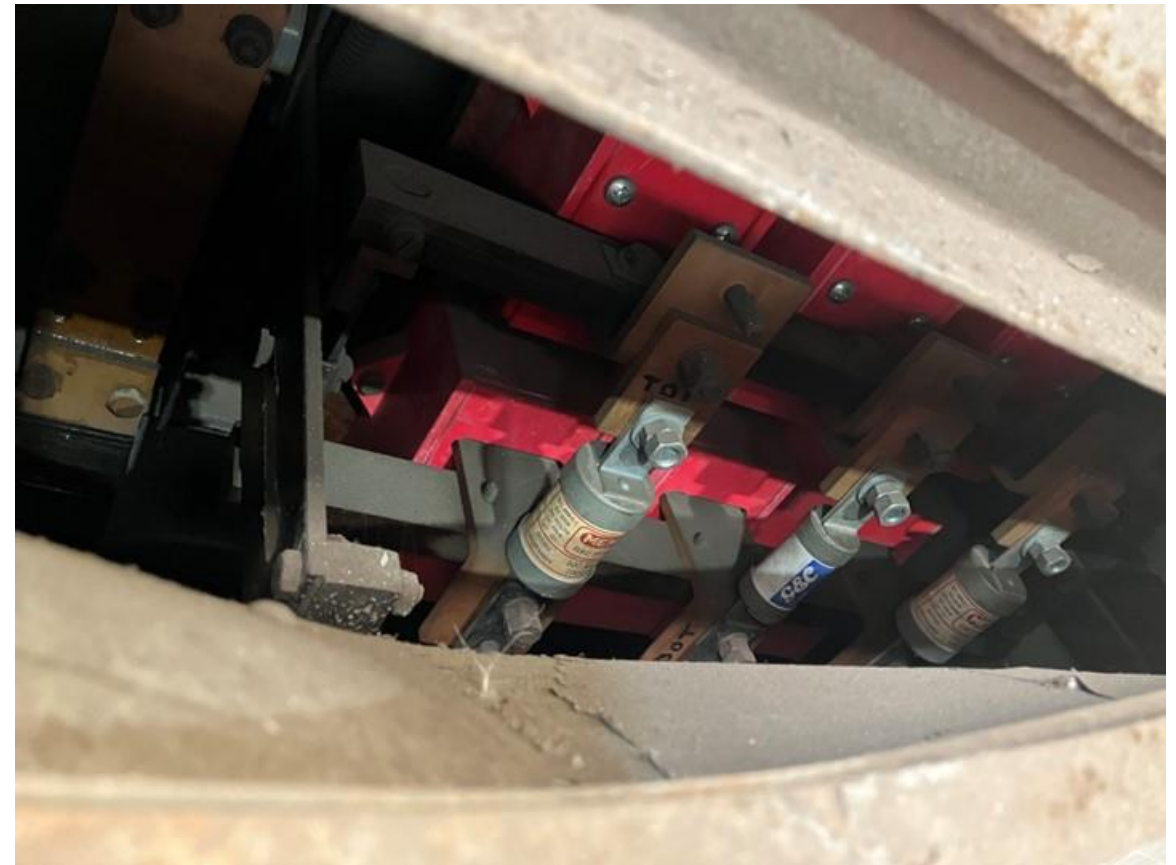
The inside view of the CFS unit through the 100mm opening. The exposed busbar and fuses are energised
