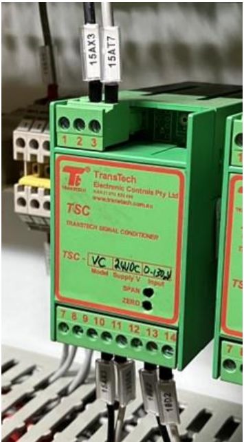
The signal isolator. Shunt wiring is on terminals 13 and 14
