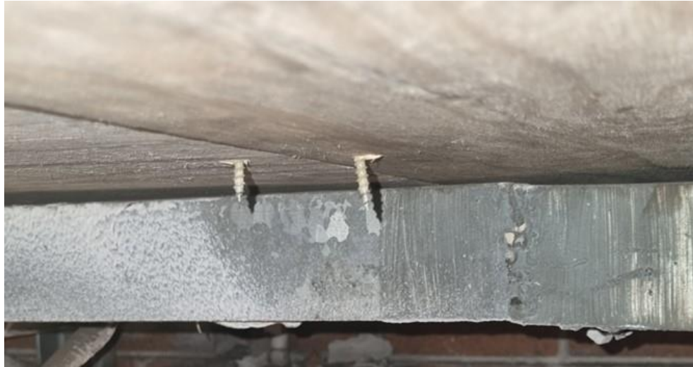
Two screws on the outside of the cable rack show the extent of penetration beyond the plyboard surface.
