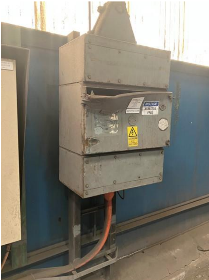
The damaged CFS unit , with door bent open and hinges sheared off
