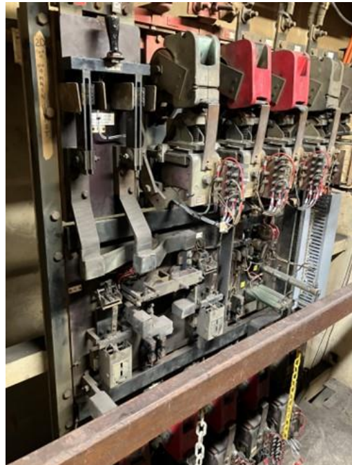
The Main Hoist DC flat back panel
