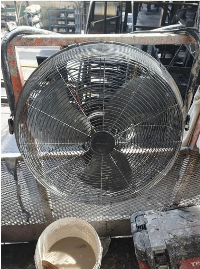
The man cooling fan secured to the hand rail of the EWP bucket fed by 240V extension lead.
