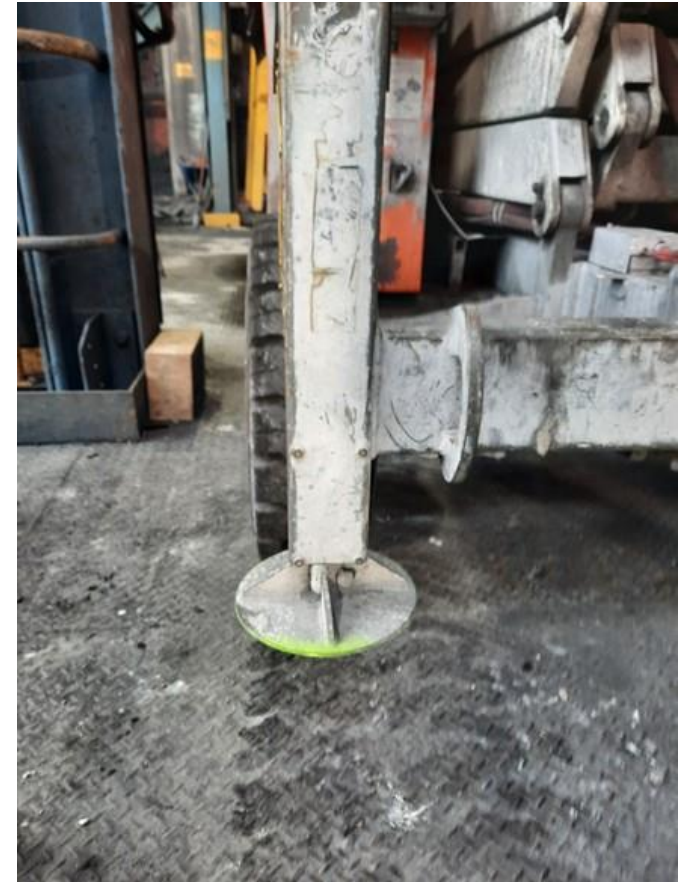
The outrigger leg of the EWP. When driven down to stabilise the EWP the foot has crushed the extension lead and explosion the conductors.
