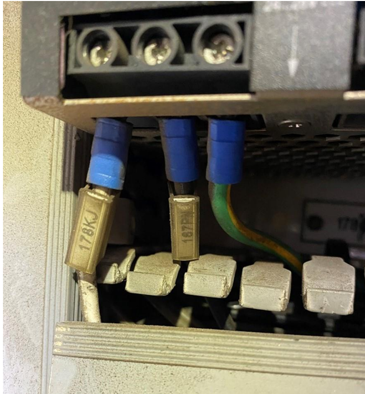
The supply terminations
