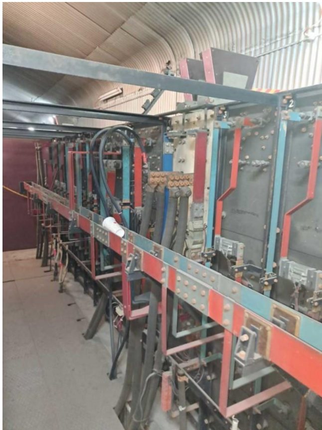
Back of DC Panels
