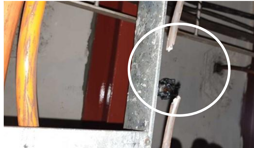
Close up of cut cable
