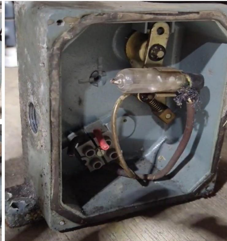
The Mercury Switch
