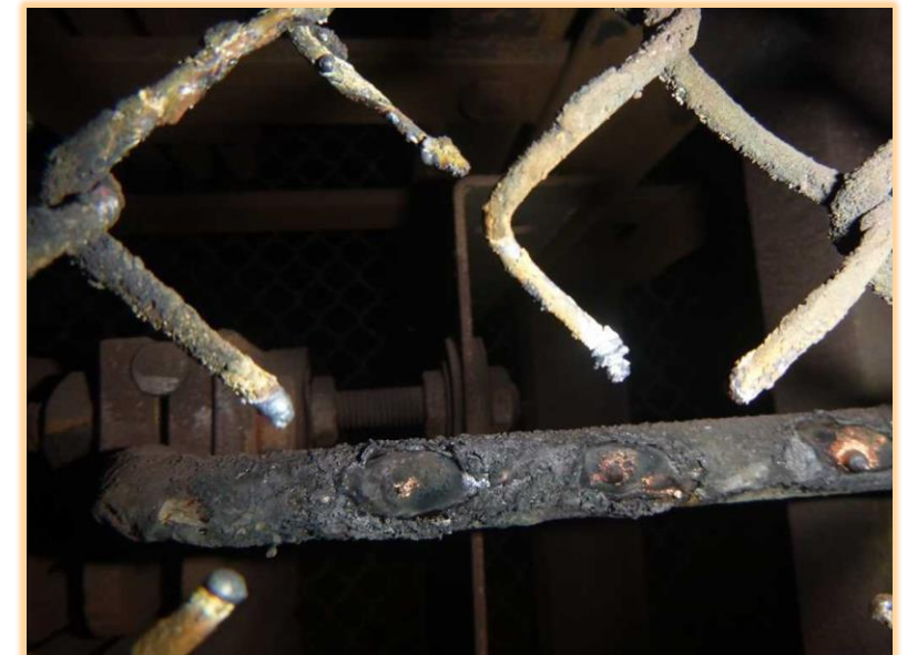
Arc marks where resistors were shorting to loose mesh
