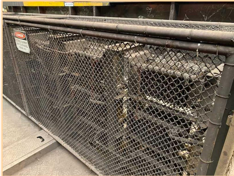
DC Crane Resistor Bank Enclosure
