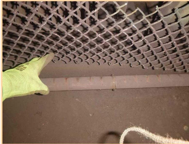
Loose Protective Mesh – wire ties broken off
