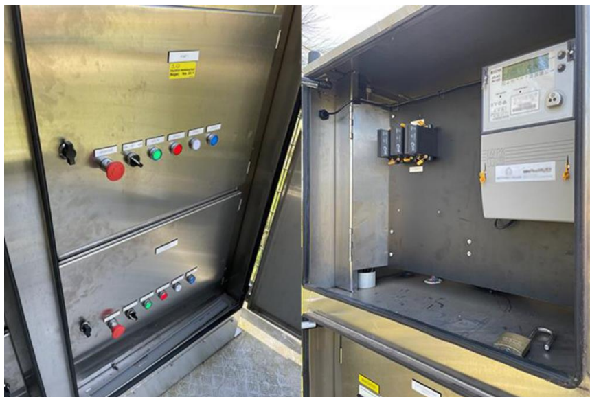
Incident site showing operator control panel that the electrical apprentice was performing work on.
